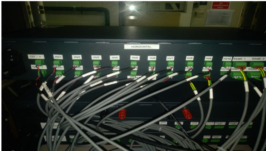
Fig. 4. MTCD2@NCBJ rear panel of the Gamma Camera. Most left connectors (label: 12V - +) are power suppliers for Filterboxes
